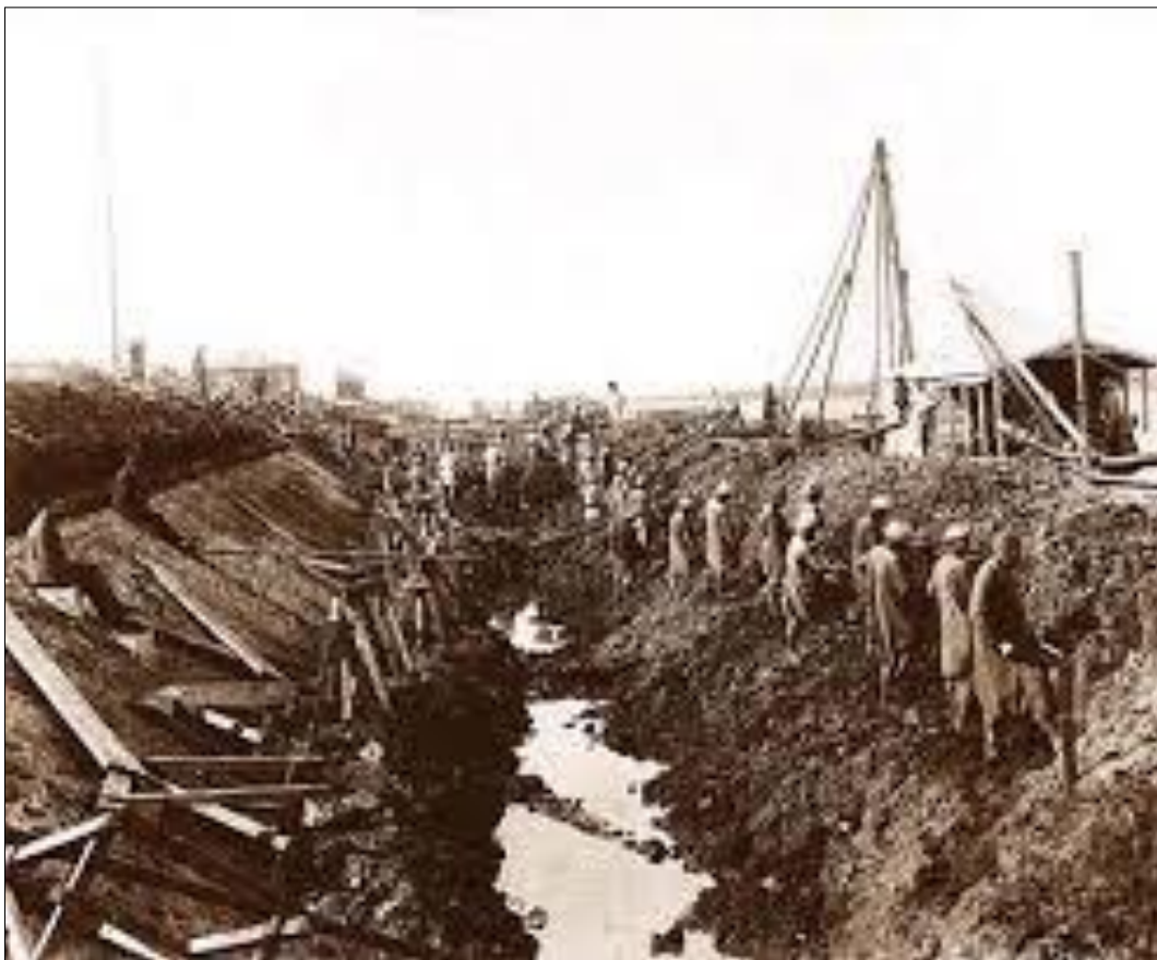
Construction of the Suez Canal began in April 1859, and at first digging was done by
