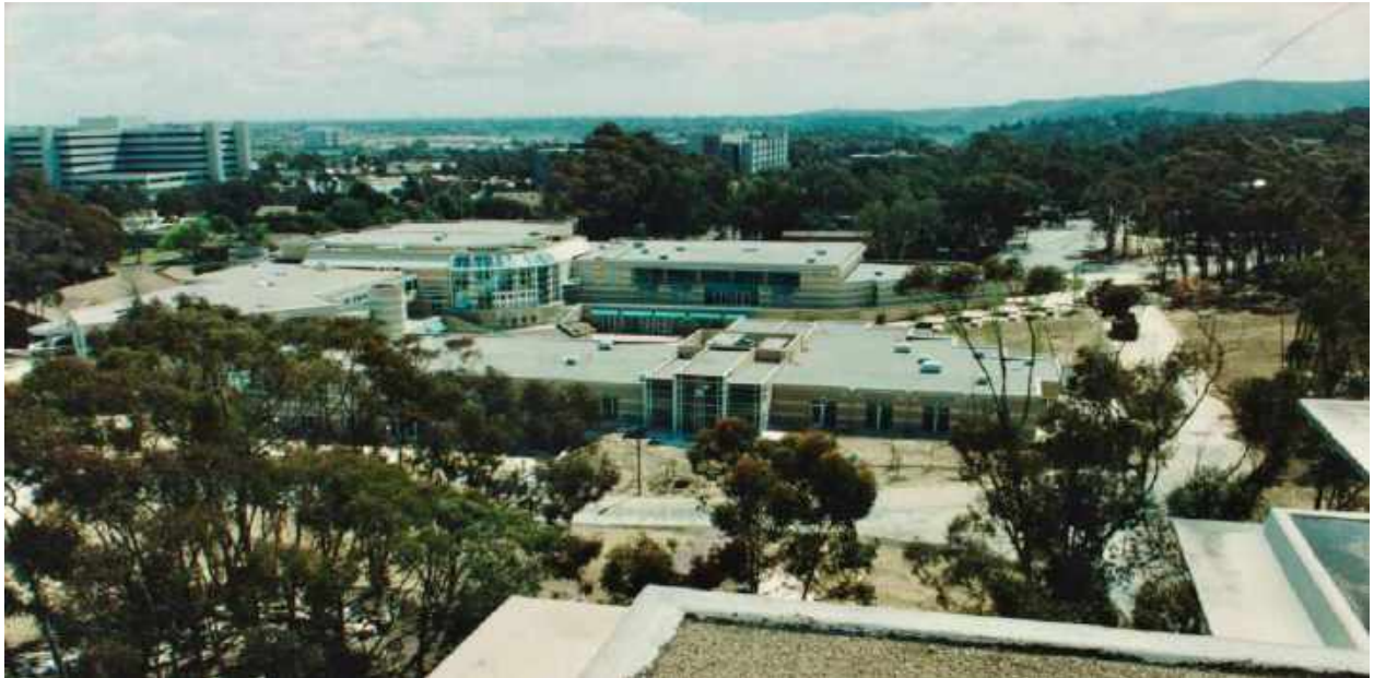
UC San Diego student union under construction, nearing completion in 1989, after I'd returned to the UK. Photo taken from the roof of William Pereira's famous library building.
