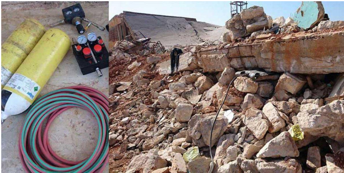
Syria airbag kit; airbag testing under collapsed building. (c) Field Ready.
