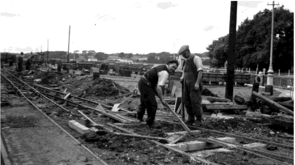
August 1954, Port Dinorwic - track relaying during the summer shutdown of the quarry
