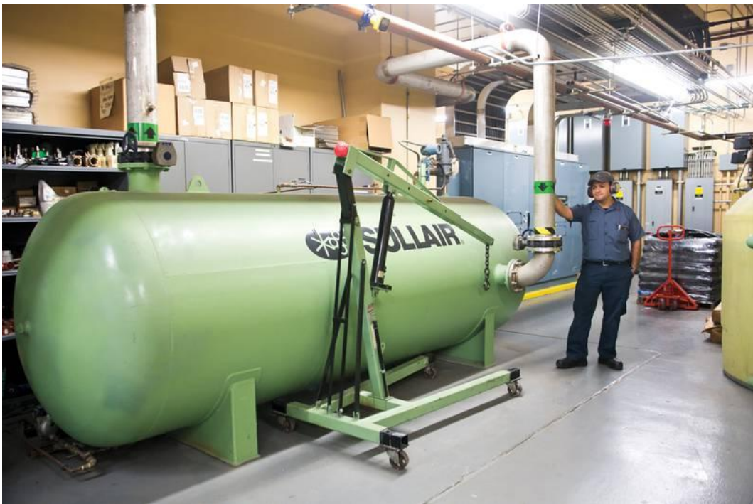
The Compressor Room beneath the Bellagio fountain.
